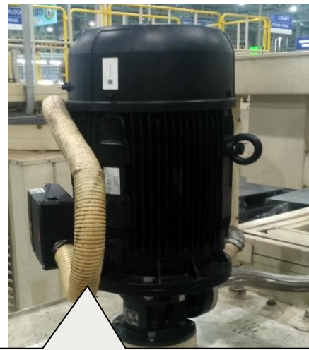
Inverter driven (Variable speed) motor- 45 Kw
