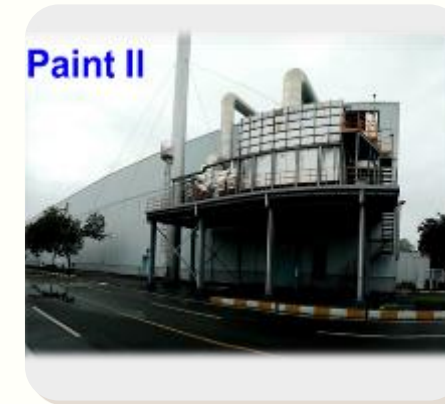
State of the art Waste heat recovery unit
